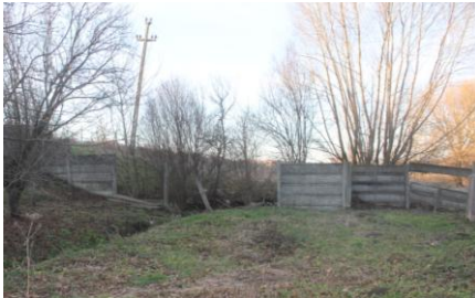
Most of the fence is broken
